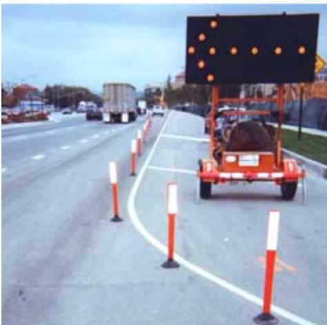
Properly placed channelizing devices and arrowboards are important in providing drivers with a clearly defined travel path.
